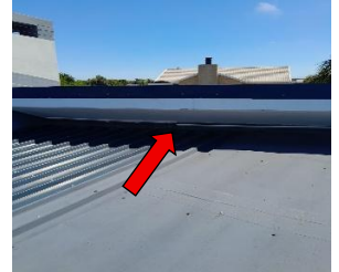
Pic 04: Damaged roof flashing and ceiling board elements.
