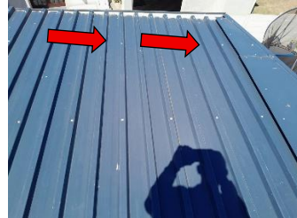
Pic 03: Deflection in metal roof sheeting.
