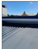
4 Damaged roof flashing and ceiling boards strips.
