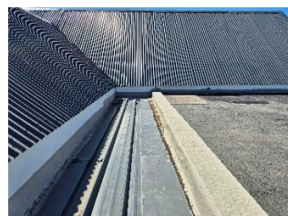
Pic 14: Flat metal sheet roof over Foyer with water leaks.
