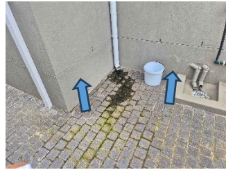
Pic 06: Water ingress/damp on external wall. Ponding water.
