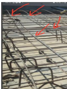
Pic 16: Top rebar bend and not fixed properly to each other.
