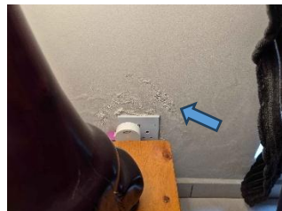
Pic 03: Water damp and paint peeling off.
