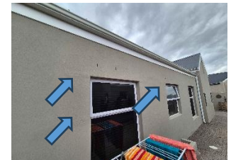
Pic 26: Horizontal cracks repaired but appear again.
