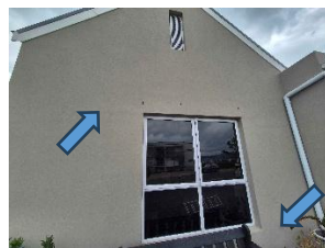
Pic 24: Horizontal cracks repaired but appear again.
