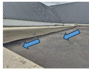
Pic 11: Garage concrete slab slopes to front with no outlet.
