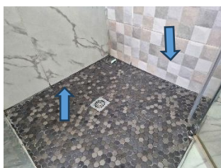
Pic 01: Poor waterproofing of the shower tiles results to leaks.
