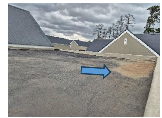
Pic 12: Ponding water with sand deposits remains.
