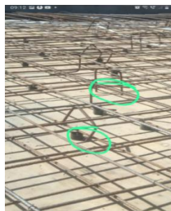
Pic 17: “Stools” installed not according to specification and trade.
