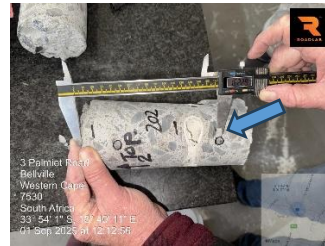
Pic 21: Core #02 – rebar located 162mm from top.
