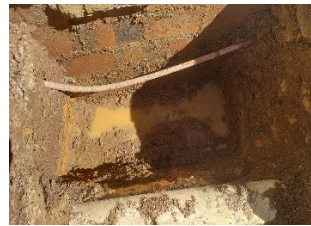
Pic 25: Test Pit #02 – standing water above foundation level
