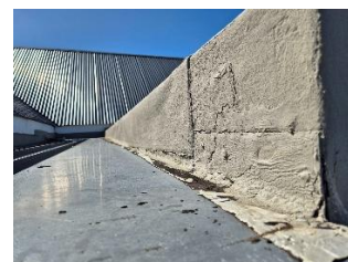
Pic 15: Flashing and waterproofing damages.
