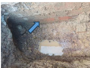
Pic 23: Test Pit #01 – water seeping from above foundation.
