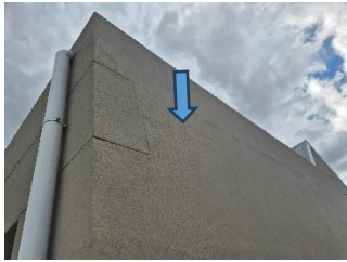
Pic 05: Water damp / ingress from garage concrete slab.
