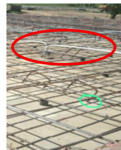
Pic18: Incorrect “stools” installed and conduit services above top steel of slab.
