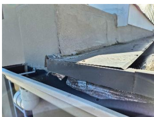
Pic 13: Damaged flashing and waterproofing. Water in gutter.
