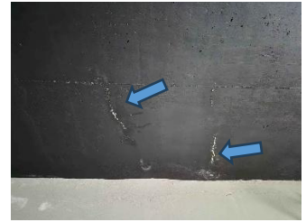
Pic 08: Water seepage and cracks in garage slab.
