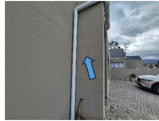
Pic 07: Rising water damp on front walls.
