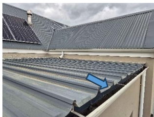
Pic 09: Little to no slope results in ponding water in the gutter.
