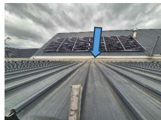
Pic 10: Back-end roof deflecting in the centre.
